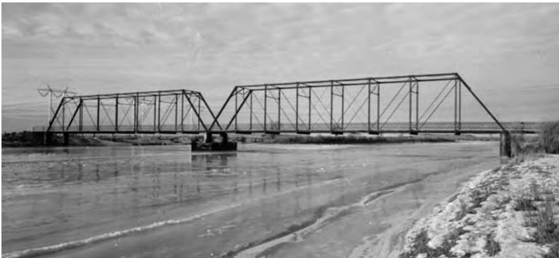
17. Big Island Bridge over Green River, County Road No. 4, Sweetwater County, WY
